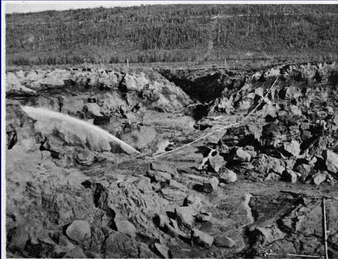
Fig. 3-3 This is a view of Cripple stripping, with pipe suspension bridge and Chena ditch visible in the background. (Boswell 1979)
